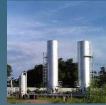
GAS FLARE SYSTEMS
